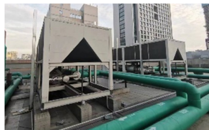
Roof-mounted air conditioning external units
