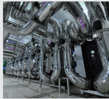
Ice storage central air conditioning
